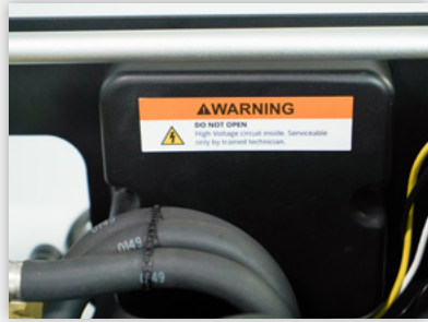
This label warns you of the residual hazards inside the WAZER Pump Box Electrical Enclosure and instructs for it to not be opened up.
